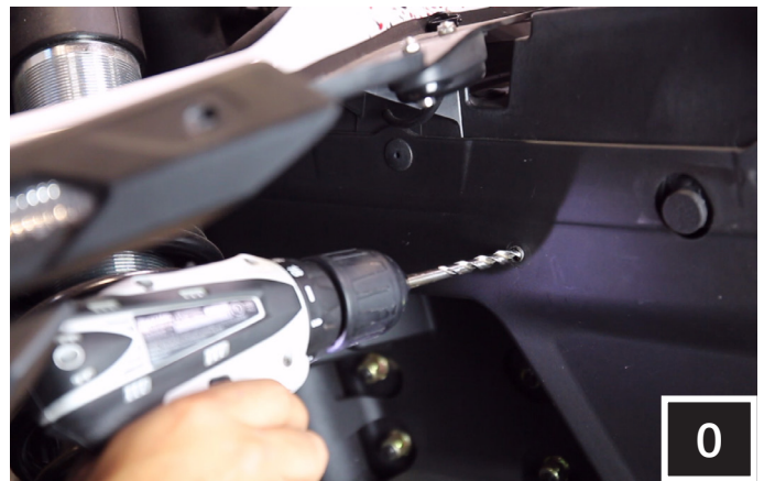
O. Drill a larger hole through the pilot hole using a 1/4" drill bit. Be sure to move the amp plate out of the way before drilling.
