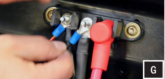
G. Run the (RED) Power and (BLACK) Ground wire of the USB/Aux input port to the Bus Bar. Unscrew the nut on the first position terminal (accessory) and attach the (RED) Power wire. Re-screw on the nut. Then unscrew the nut on the second position terminal and attach the (BLACK) Ground wire. Re-screw on the nut.
